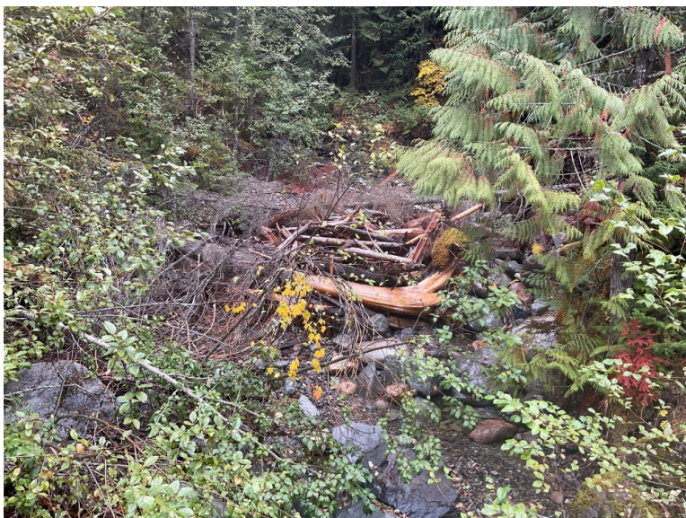
Debris accumulation upstream
