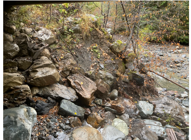
Riprap erosion downstream left bank
