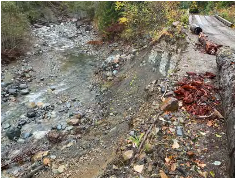
Left bank approach fill slope severely eroded
