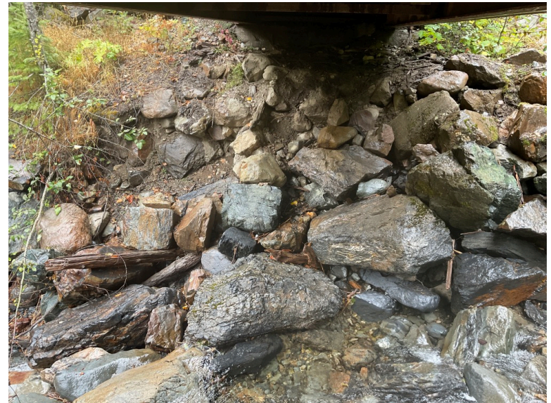
Riprap erosion at right bank
